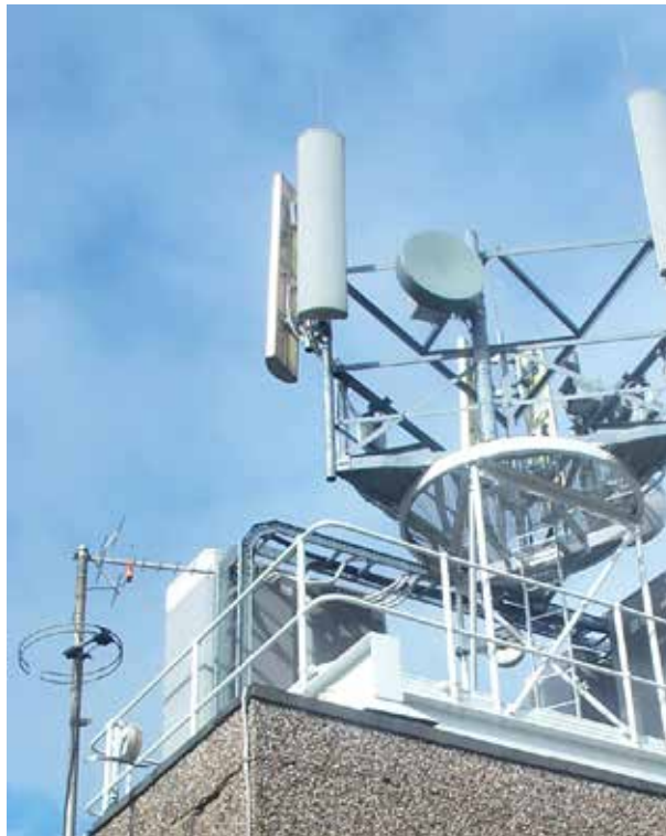
Figure 10.1 — Mobile phone sector antennas and a microwave dish on the roof of the lift house
