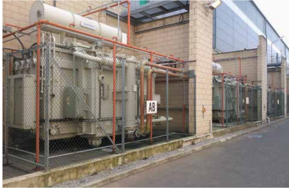
Figure 3.4 — The transformer bays
