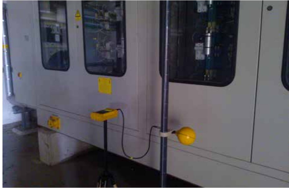
Figure 3.6 — Measurements being made near a thyristor rectifier
