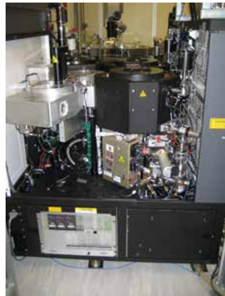
Figure 9.2 — Reaction chambers in the service area
