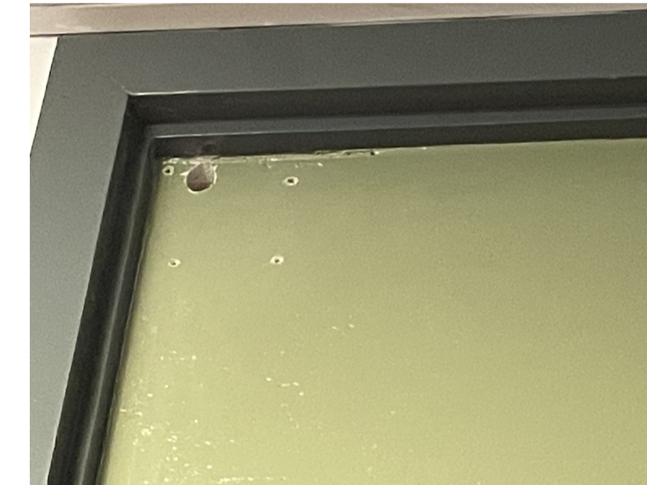
Existing Door hole to be repair or replaced to keep the door 60 minute fire resistance
