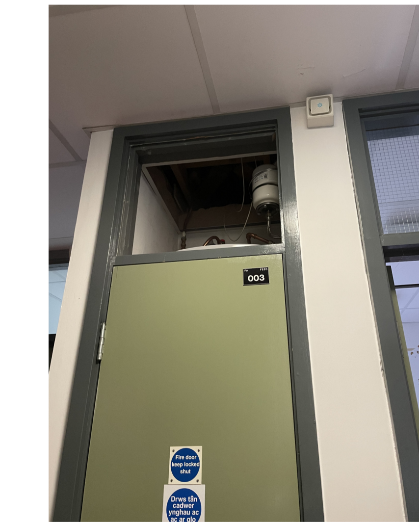
Missing over panel, new 60/60 panel to be replaced by 60 mins integrated and insulated. Ventilation requirement to be confirmed by MEP. Missing ceiling above and above void. Input from fire consultant required.
